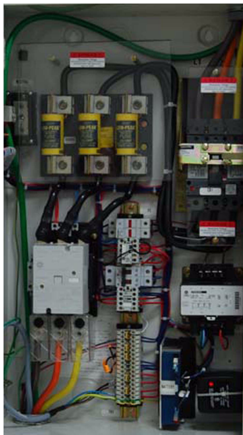
Figure 14-1 Primary Power Disconnect (A1)
